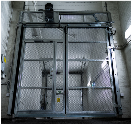
Double doors with lock function and recessed access door for emergency evacuation.
